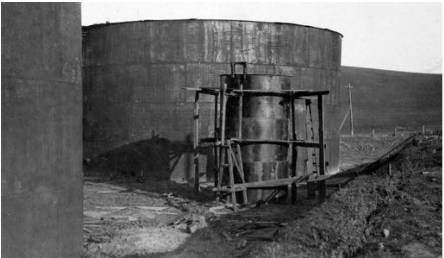
Placing boiler in Wharf Boiler House, from north end of building. View looking west. January 19, 1913.
