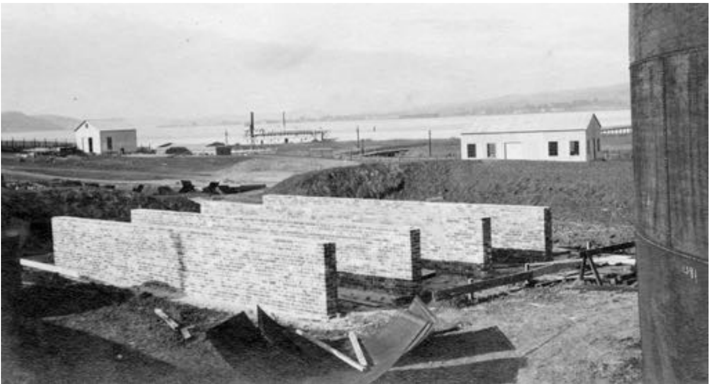
Service tanks foundation completed with Boiler House, ferry boat 'Onward', wharf approach and Filling Shed in distance. Edge of Tank #5 far right. View looking West. January 2nd, 1913
