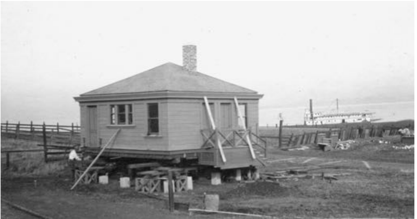
Office Building as side of road ready to be lowered unto its foundation. October 23rd, 1912.
