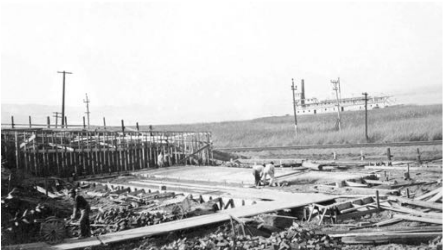
View looking North West. Retaining wall being constructed behind new Dormitory foundation under construction. Old ferry 'Onward' in background. November 11th, 1912.
