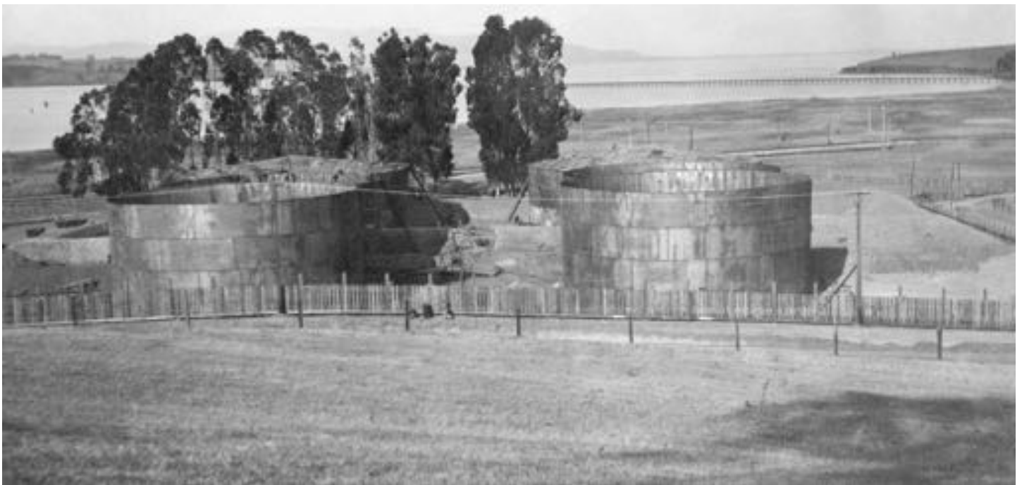
Roofs being installed on Tank #1 and #2. Tank#5 and #6 by road at sharp bend. American Occidental refinery wharf in distance. View looking north. December 15th, 1912
