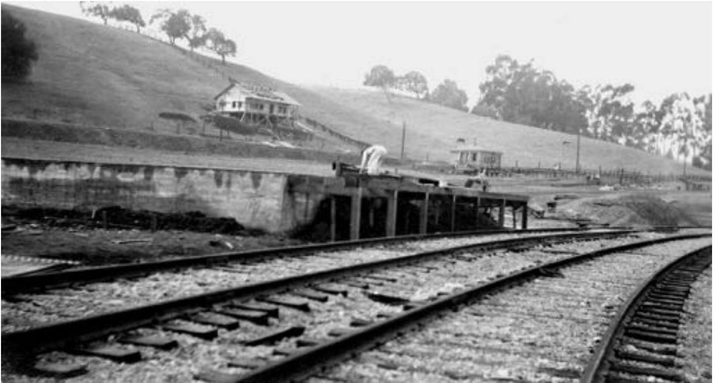
Filling Shed and dock under construction beside tracks. Manager's Bungalow under construction and new office building in background in final position. October 23rd, 1912.
