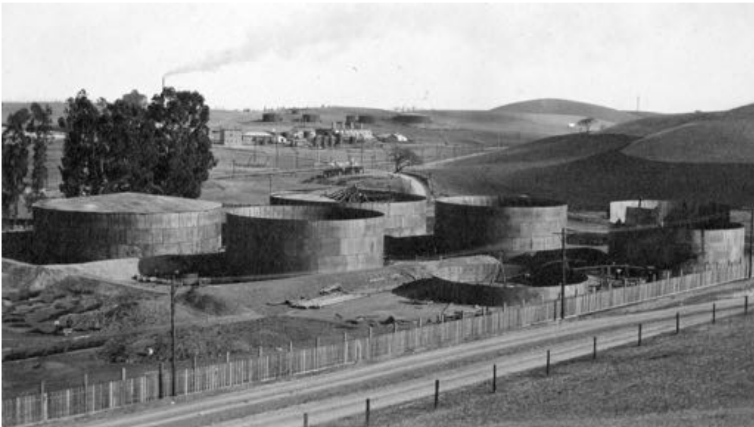
The six tanks in various stages of construction. Tank #1 with roof being installed, Tanks #3 & #4 ready for roof, Tanks #5 & #6 with sides still being erected. View looking North East. December 5th, 1912
