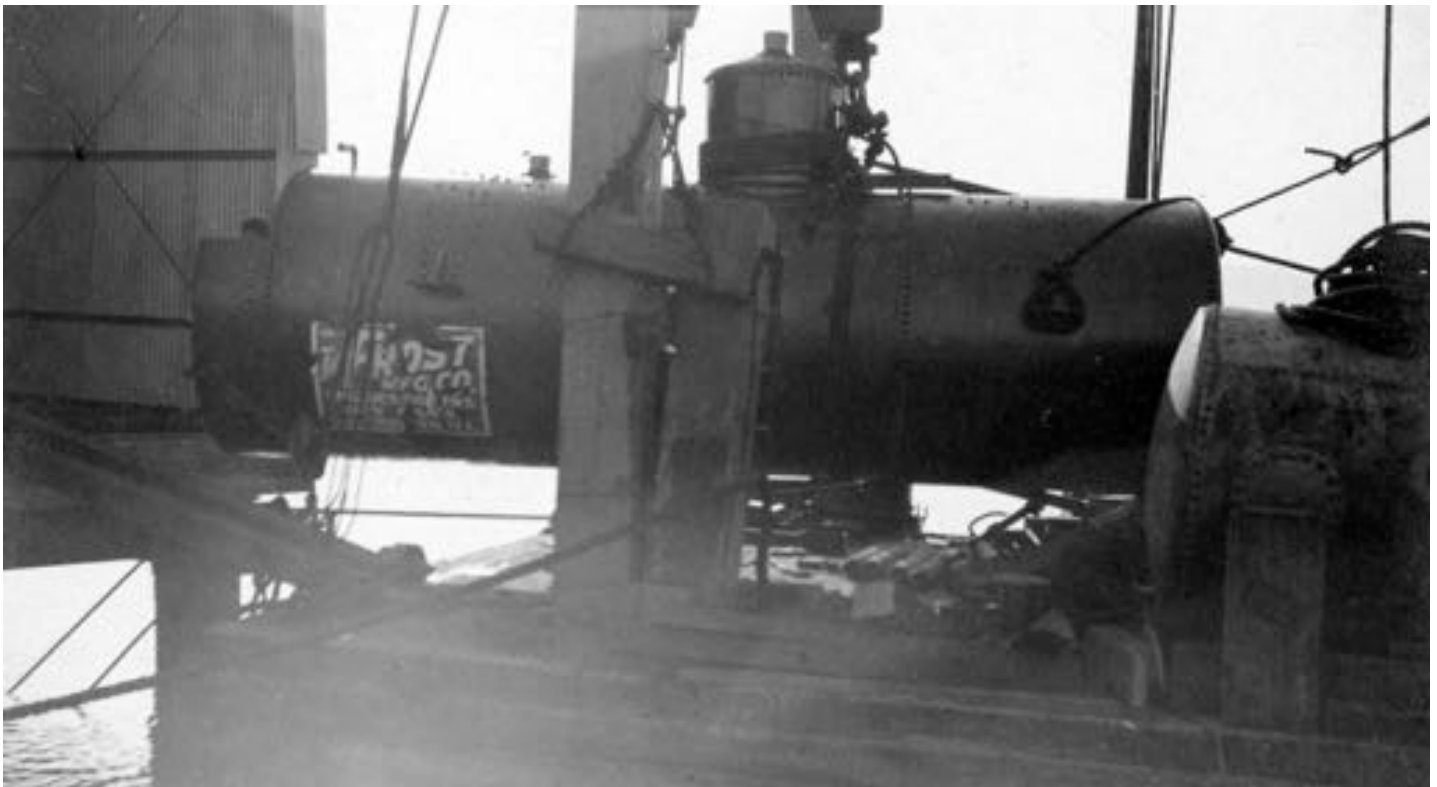
Placing boiler in Wharf Boiler House, from north end of building. View looking west. January 22, 1913.
