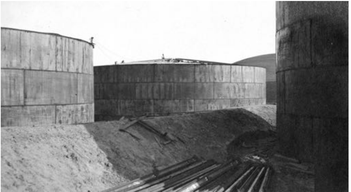
Piping being installed between Tanks #1, #2 & #3. Tanks under construction. View looking North East. December 5th, 1912
