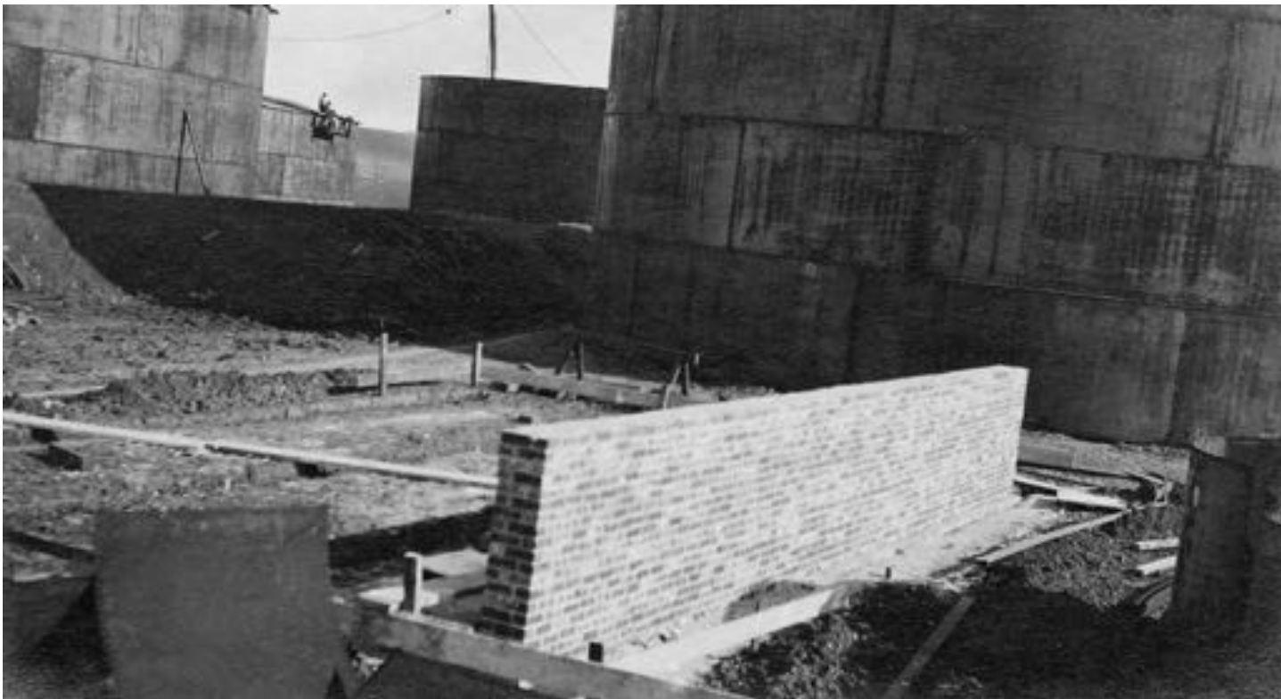
Beginning construction of foundation for 10' x 30' Service Tanks . View looking East. December 21st, 1912
