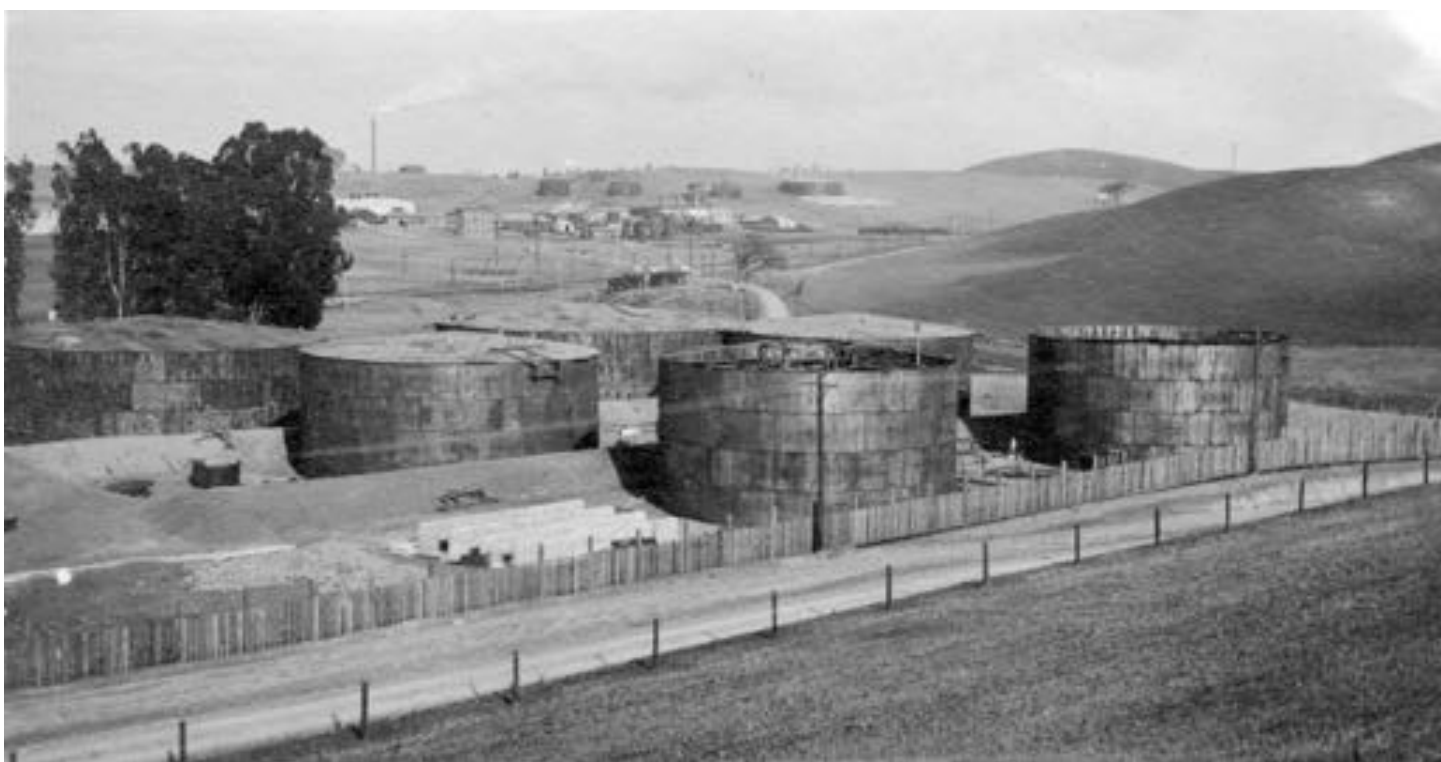
The six tanks in various stages of construction. Tank #1 thru #4 with roof installed, Tanks #5 & #6 ready for roof. Service Tanks foundation completed. The American Oriental Company refinery in the background and the smoke stack of Mountain Cooper smelter. December 27th, 1912
