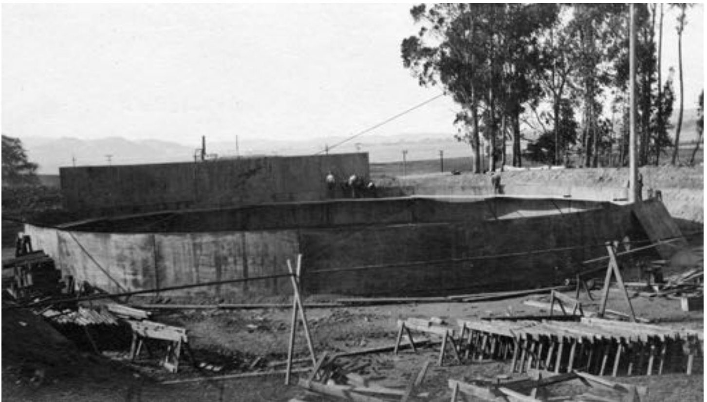
Tank #1 under construction. Second pass of tank side being installed. Wood "horses" in foreground were used to raise bottom off ground for riveting. View looking North West. October 23rd, 1912
