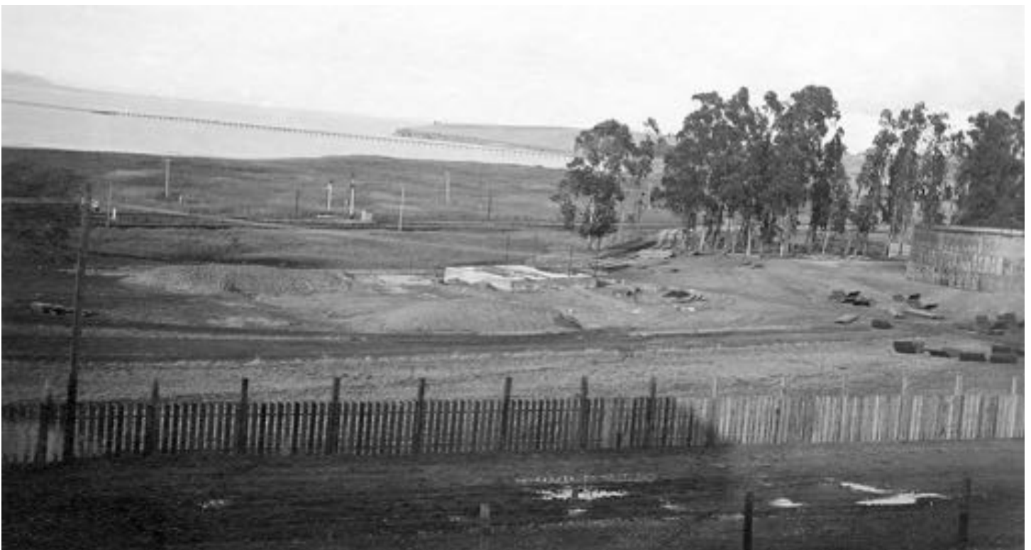
View looking North. Filling Shed foundation under construction by railroad siding. Edge of Tank #1 far right. Long Wharf of the American Oriental Refinery in back ground. November 10th, 1912.
