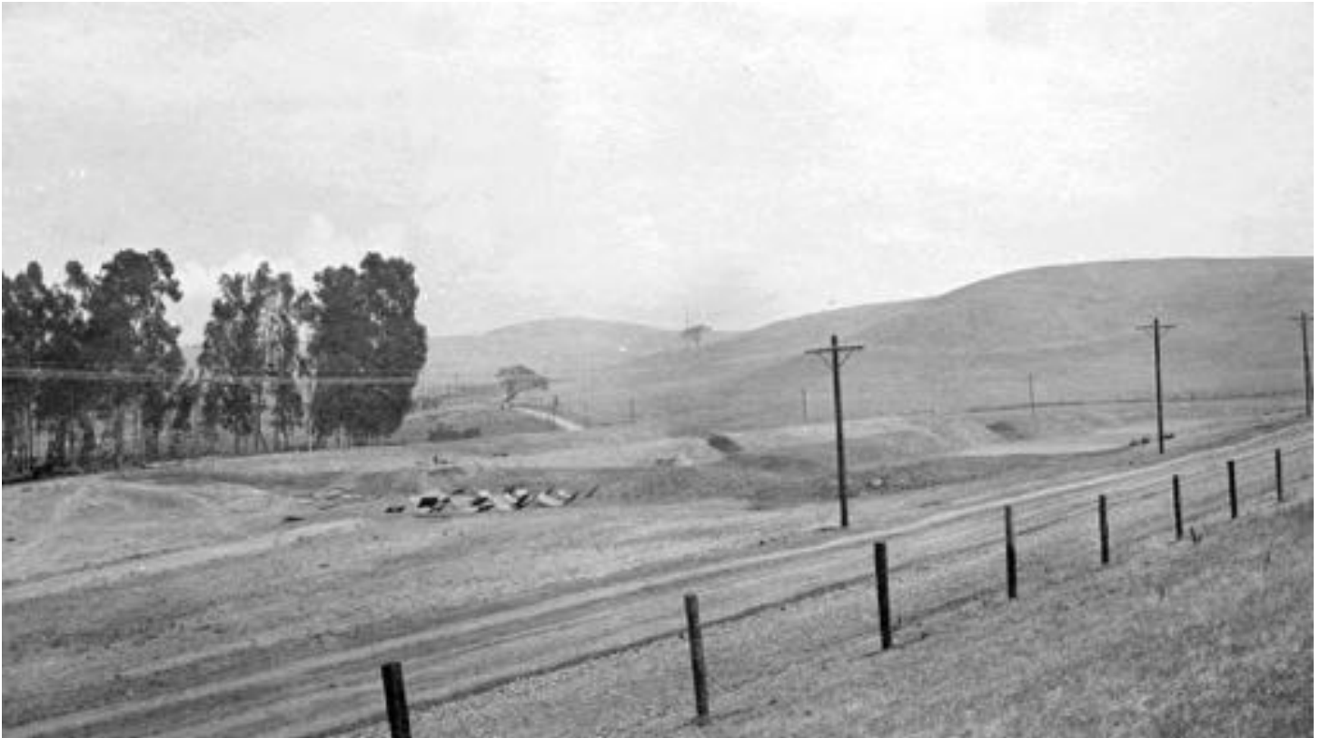
Area graded for tanks. Material for tank on ground with tank #1 under construction inside earthen banks. View looking north east with Marina Vista road behind wire fence. September 27th, 1912
