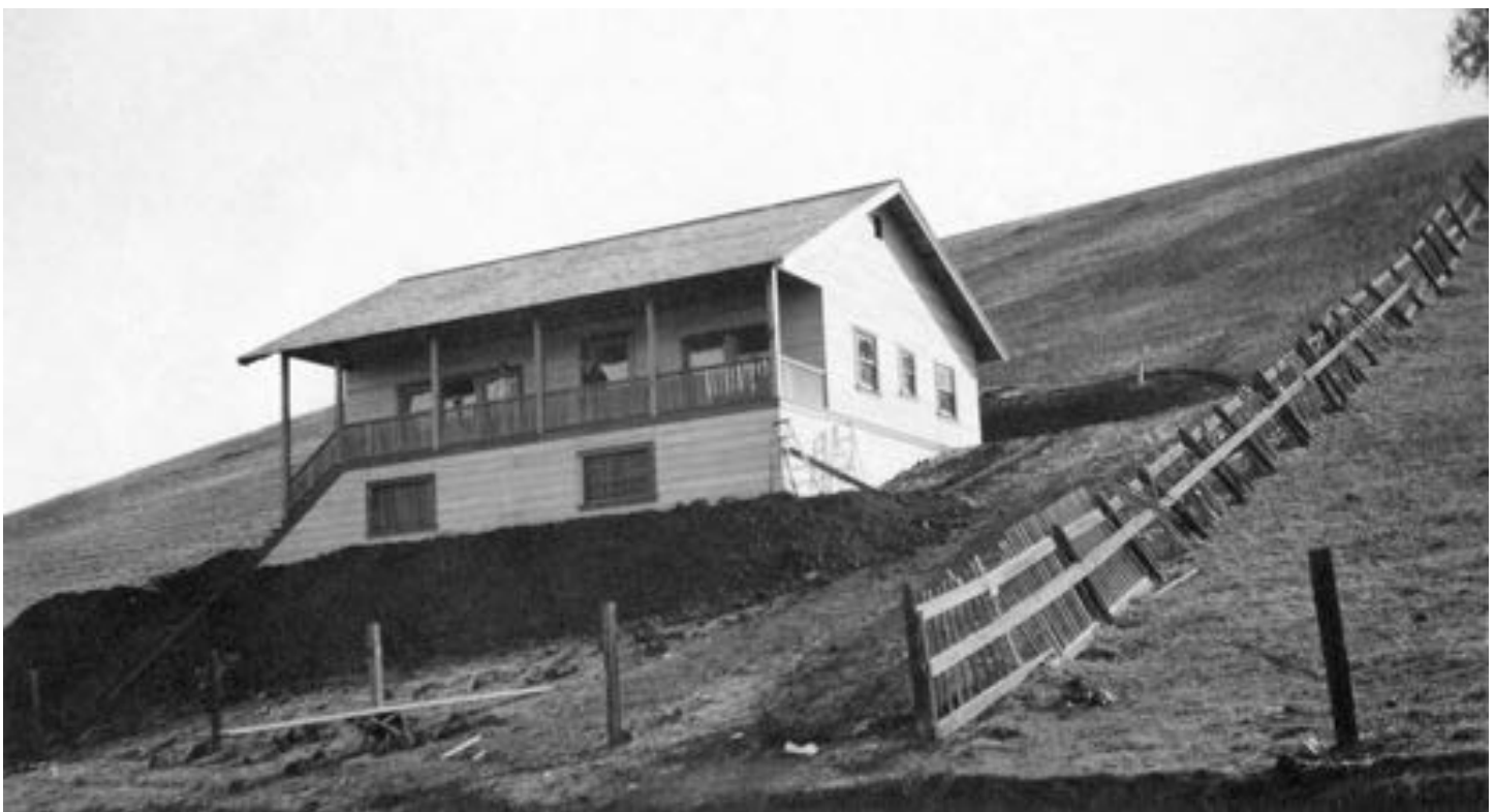
Bungalow nearing completion across road from office. View looking South East. November 11th, 1912
