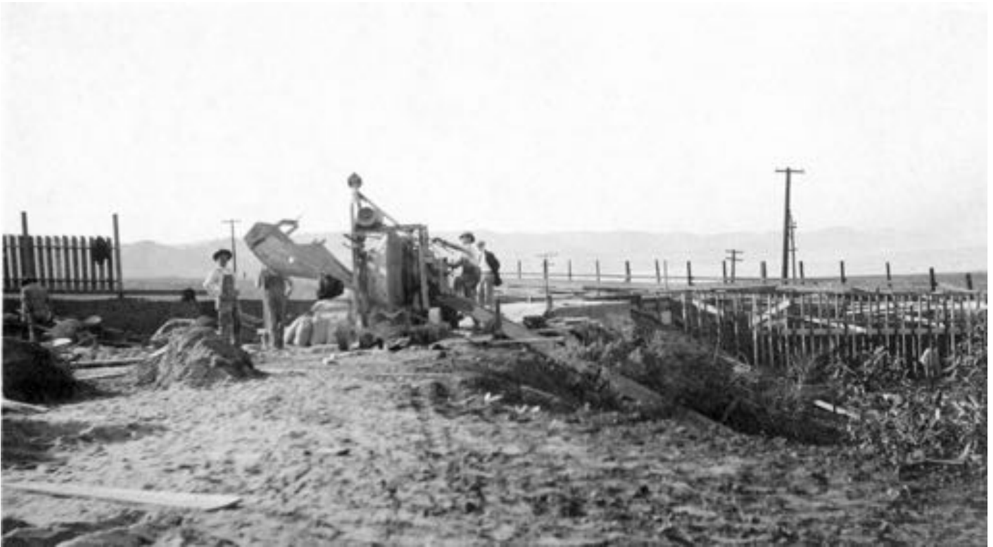
Concrete Mixer next to future 30' x 30' boiler house. View looking West. November 11th, 1912
