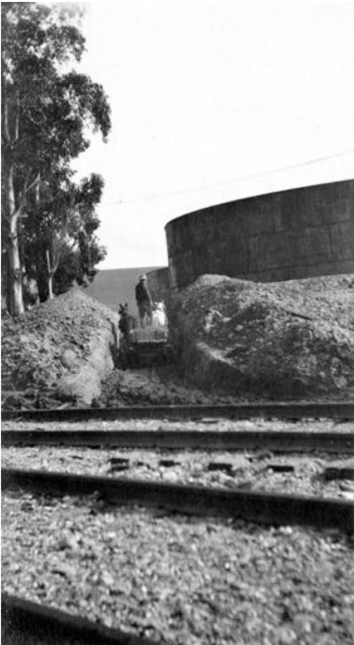
Left:: Building the run for the main Pipe lines behind tanks #1 and #2. View looking east. January 24th, 1913.
