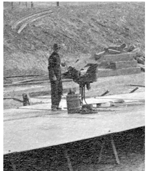
Detail of from above and from image on page 9 of man at forge getting ready to heat rivets for the fabricating of tank bottom.
