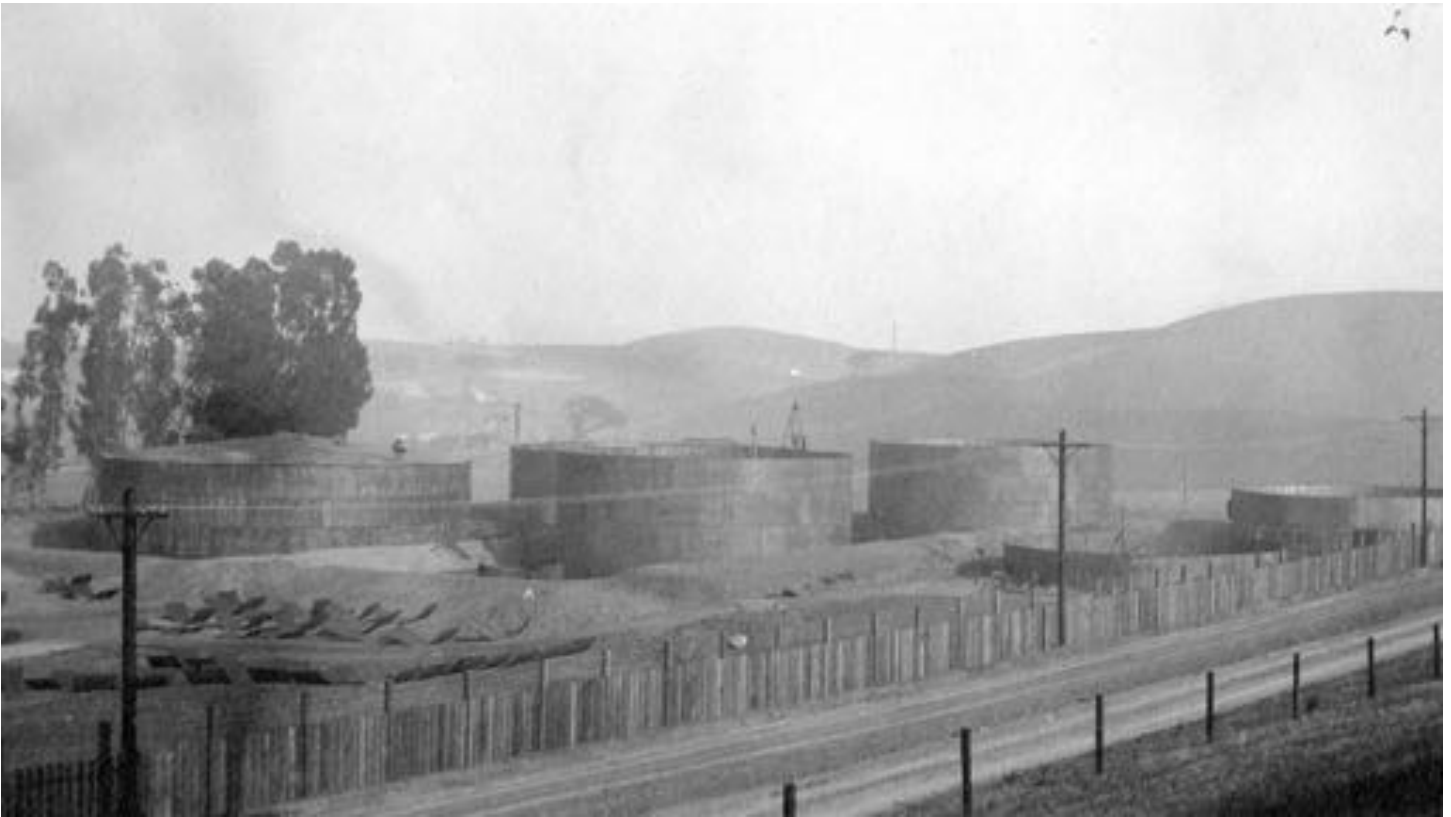
The six tanks in various stages of construction. Tank #1 with roof installed, Tanks #2, #3 & #4 ready for roof, Tanks #5 & #6 with sides still being erected. View looking North East. December 1st, 1912
