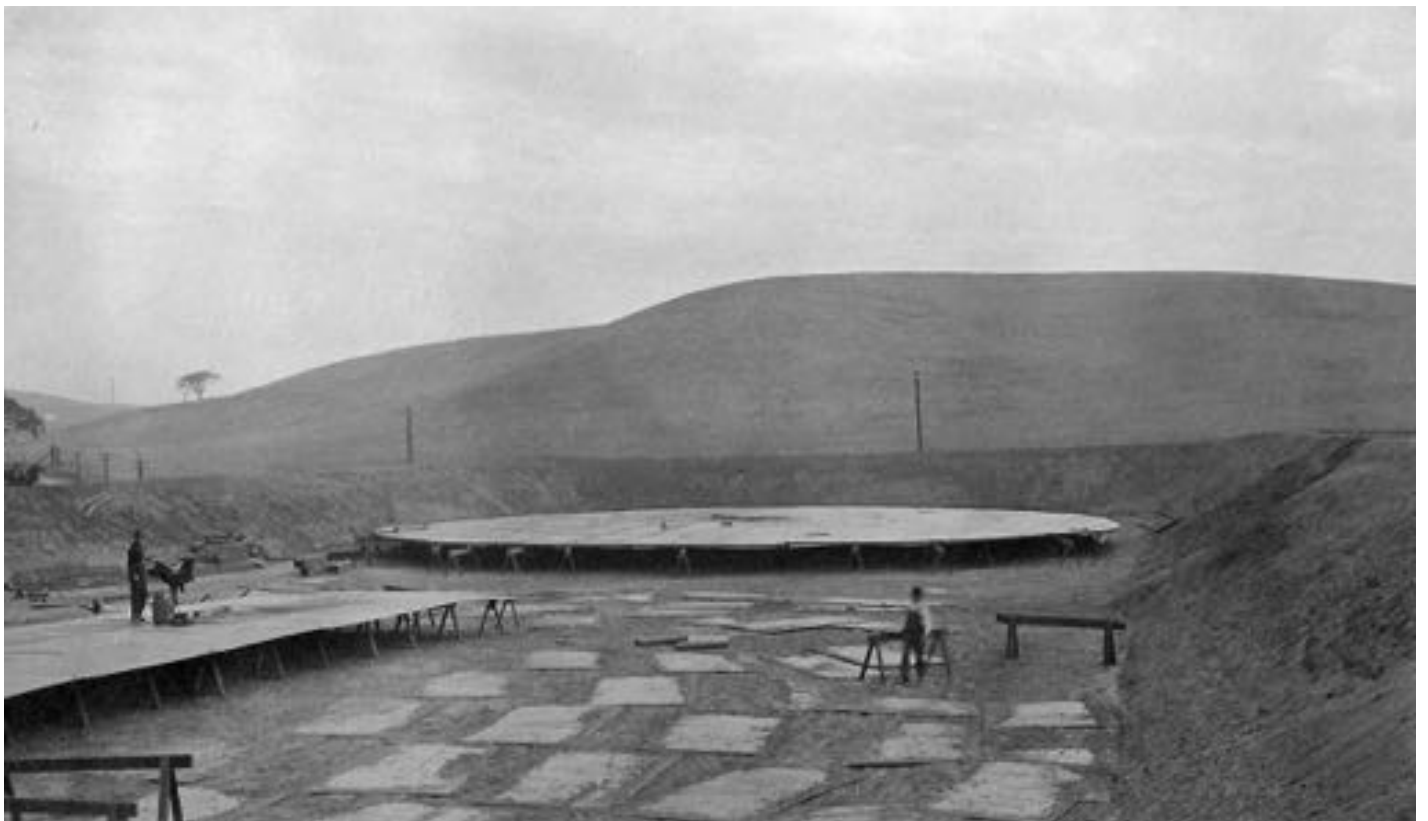
View of tank bottom #2, 95' 6" diameter completed. Tank #1 bottom under construction with bottom plates spread out on the ground. Man to the left heating rivets for construction of bottom. September 22nd, 1912
