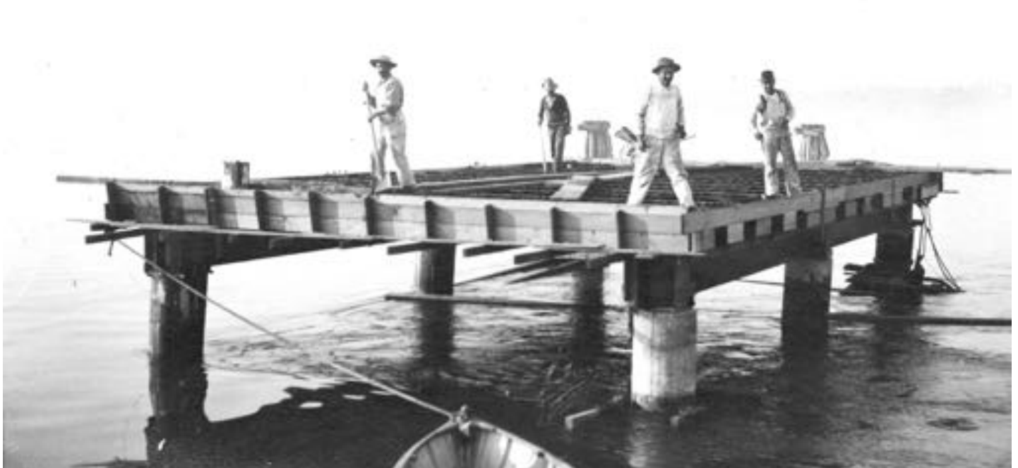
25 ft x 45 ft Boiler House foundation on piles on the west side of wharf. View looking north. October 16th, 1912.
