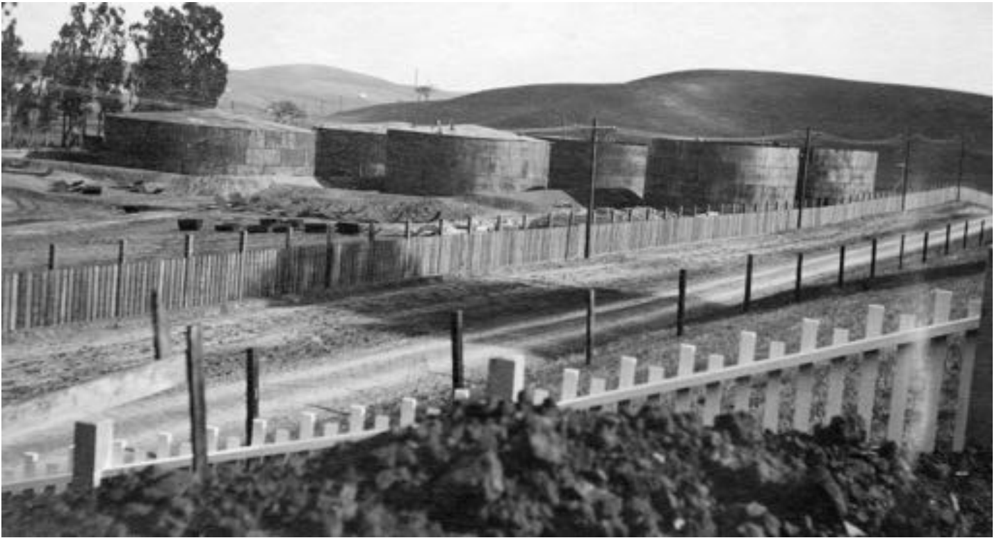
Tanks #1 thru 6 nearing completion. Roofs being installed. View looking North East. December 21st, 1912
