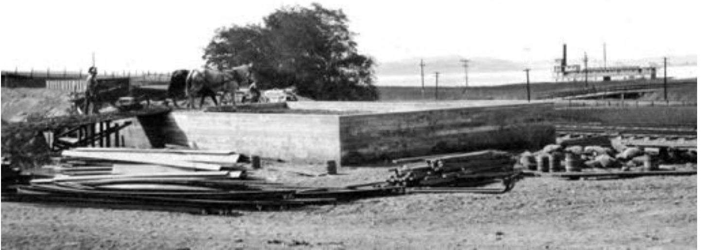
Filling Shed under construction being filled with soil. Railroad siding tracks just behind foundation and road in foreground. View looking North West. October 16th, 1912
