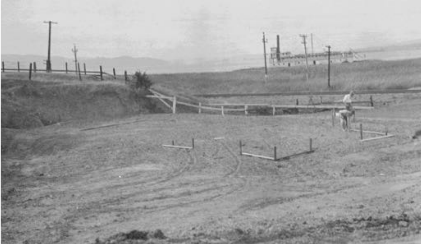
Start of construction of Dormitory staking out foundation. View looking North West. September 30, 1912.
