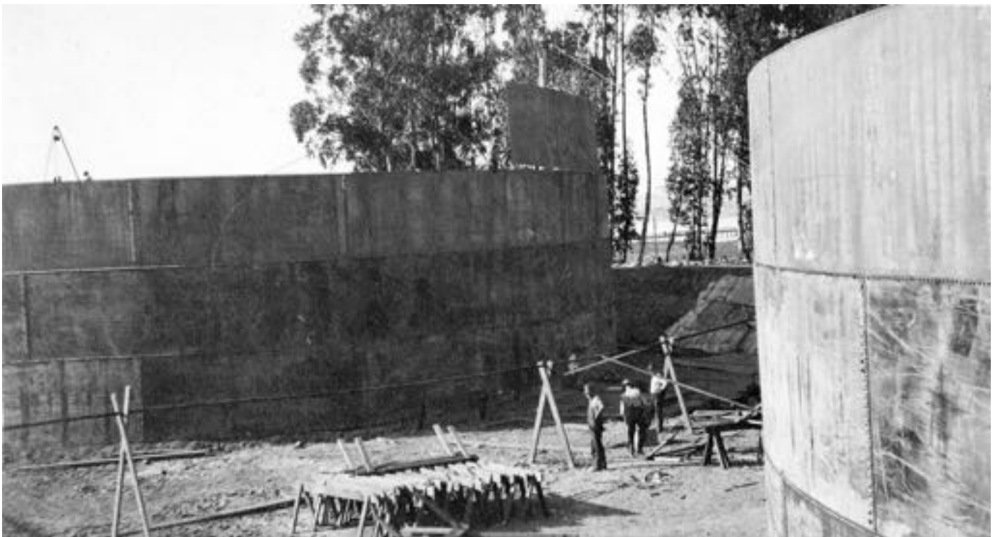
Tank #1 left & #2 right under construction. Tank #1 having fourth pass of side installed. Pipe across between the tanks above the workers is an air line for the rivet hammer. View looking North East with wharf of the American Oriental Company through trees. October 30th, 1912
