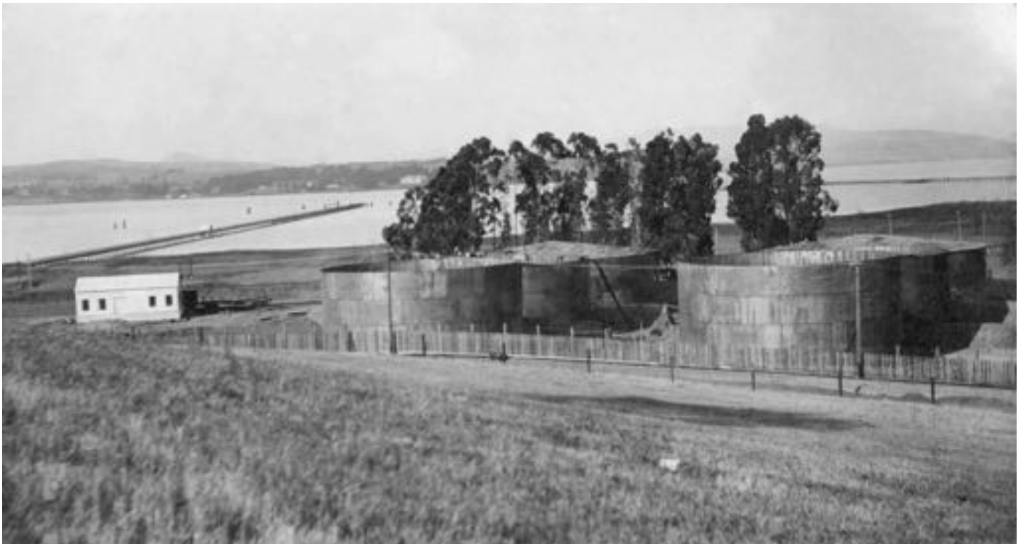
Wharf and Filling Shed left of tanks nearing completion with roofs being installed. Tanks #5 and #6 close to road. View looking north west. December 15th, 1912
