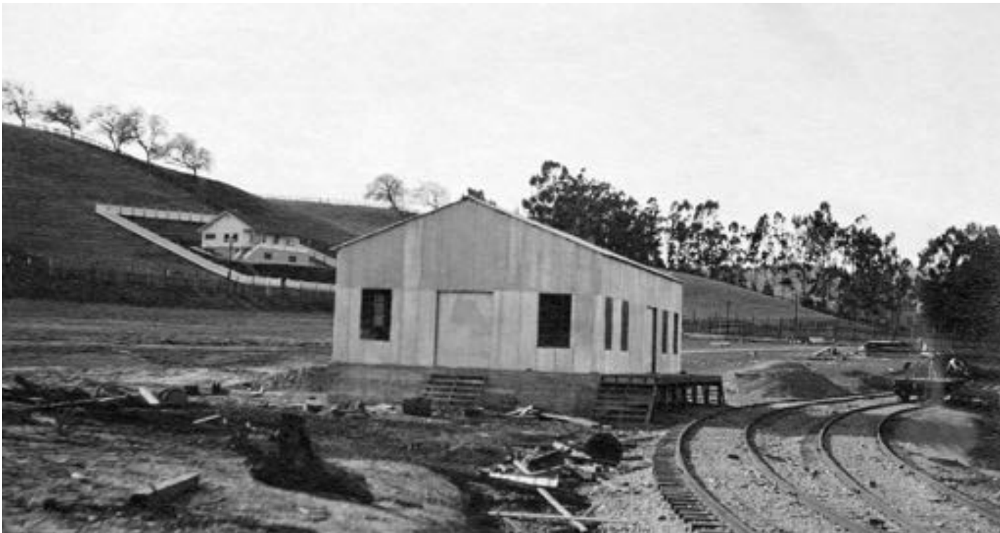
Filling Shed with railroad spur. Bungalow nearing completion. View looking South West. December 21st, 1912.
