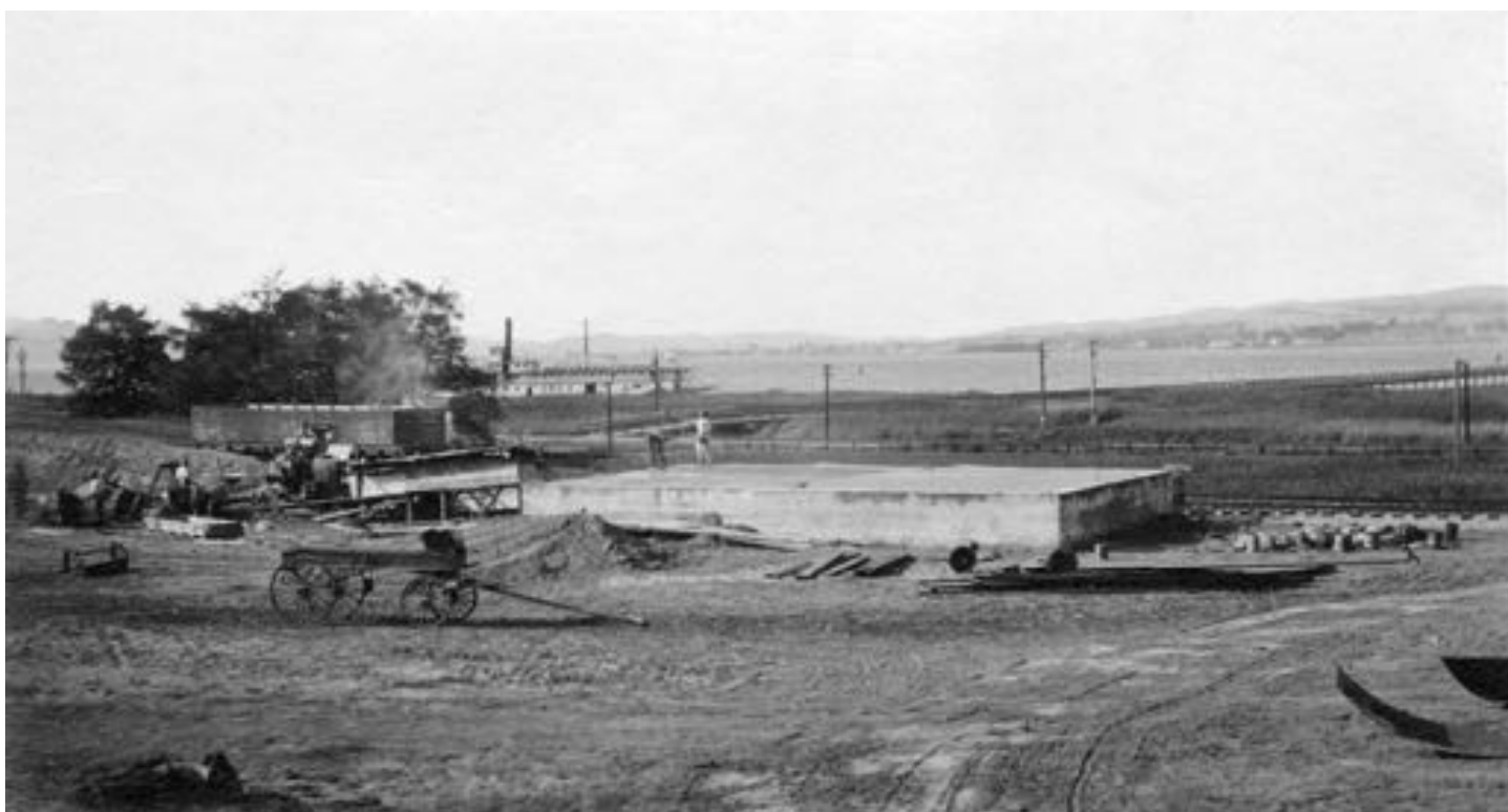
Cement mixer at Filing Shed pouring floor for Shed. Land end of Wharf in background to right. October 23rd, 1912
