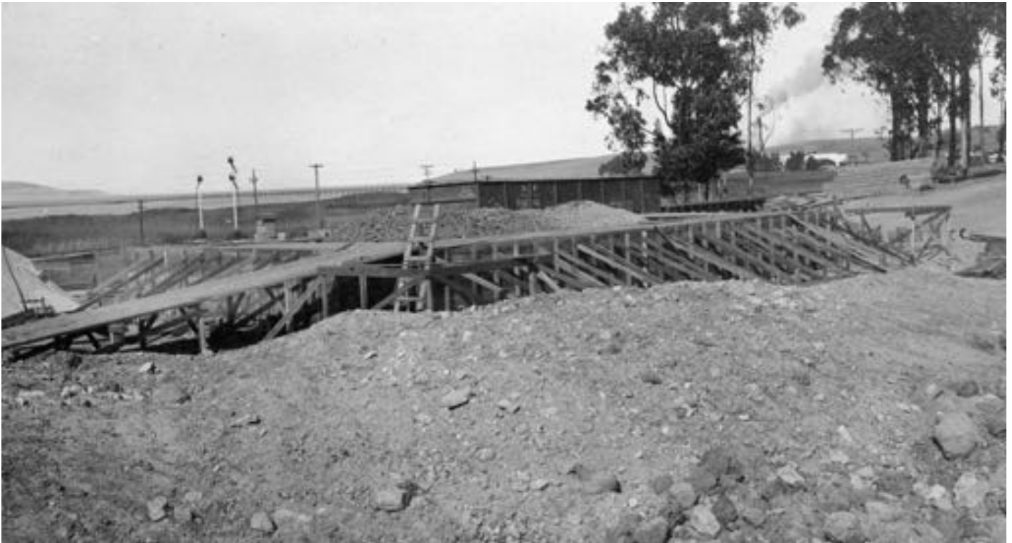
Foundation of Filling Shed ready getting ready for concrete. Gondola car on railroad siding. View looking North East. October 8th, 1912
