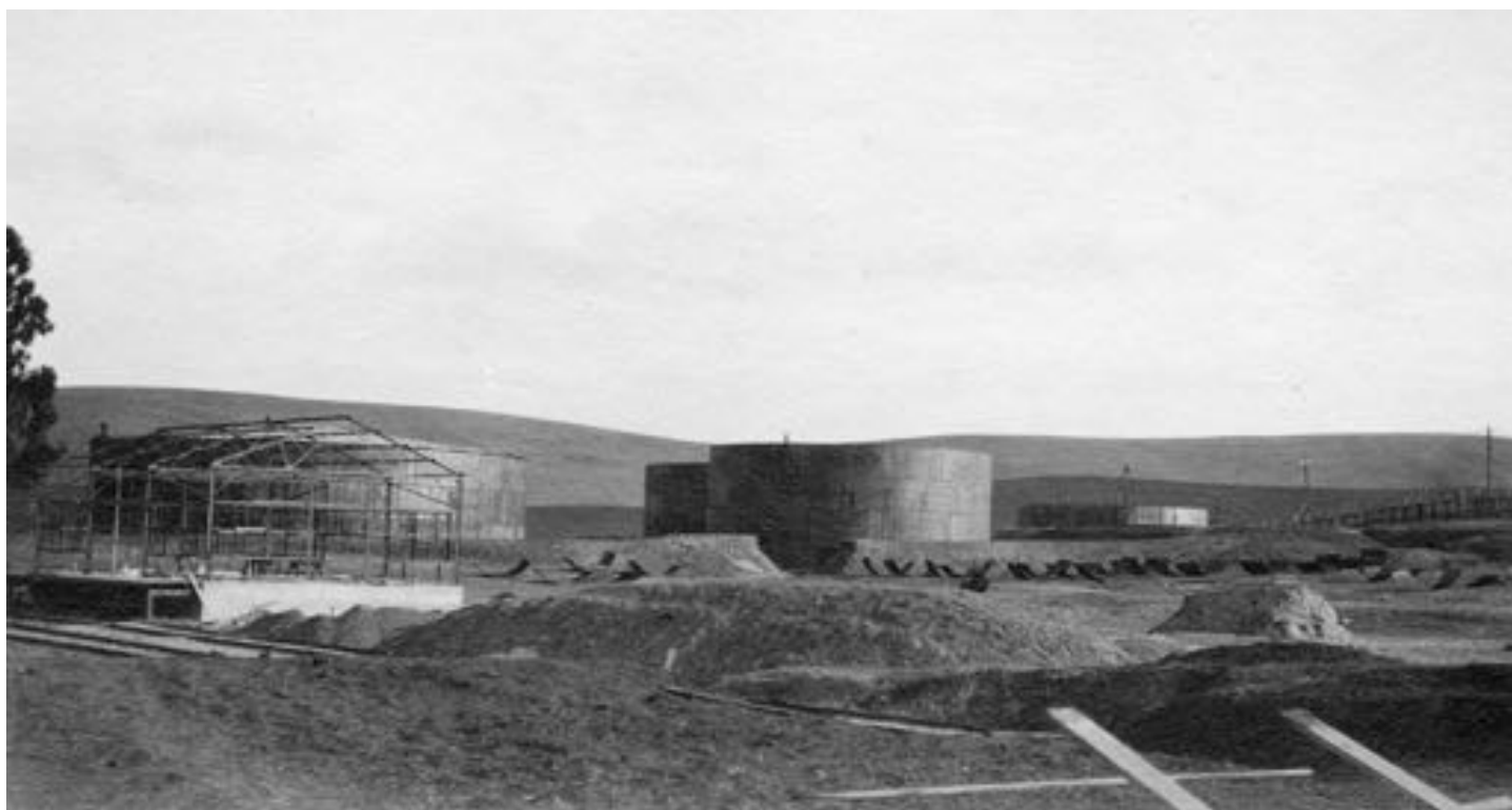
Filling Shed under construction. Tanks #1 with roof, Tanks #2 thru #6 in various stages of construction. View looking East. Empty hill in background to be location of future refinery in 1915. December 1st, 1912
