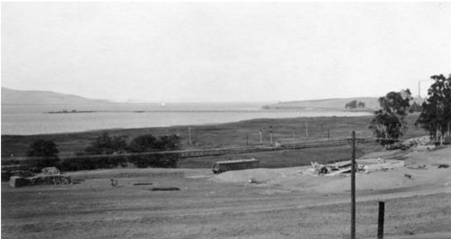
View looking North East from fence. Filling Shed foundation under construction to right, railroad siding with open boxcar to left of shed foundation on siding. The American Oriental Refinery Wharf in distance. October 23rd, 1912
